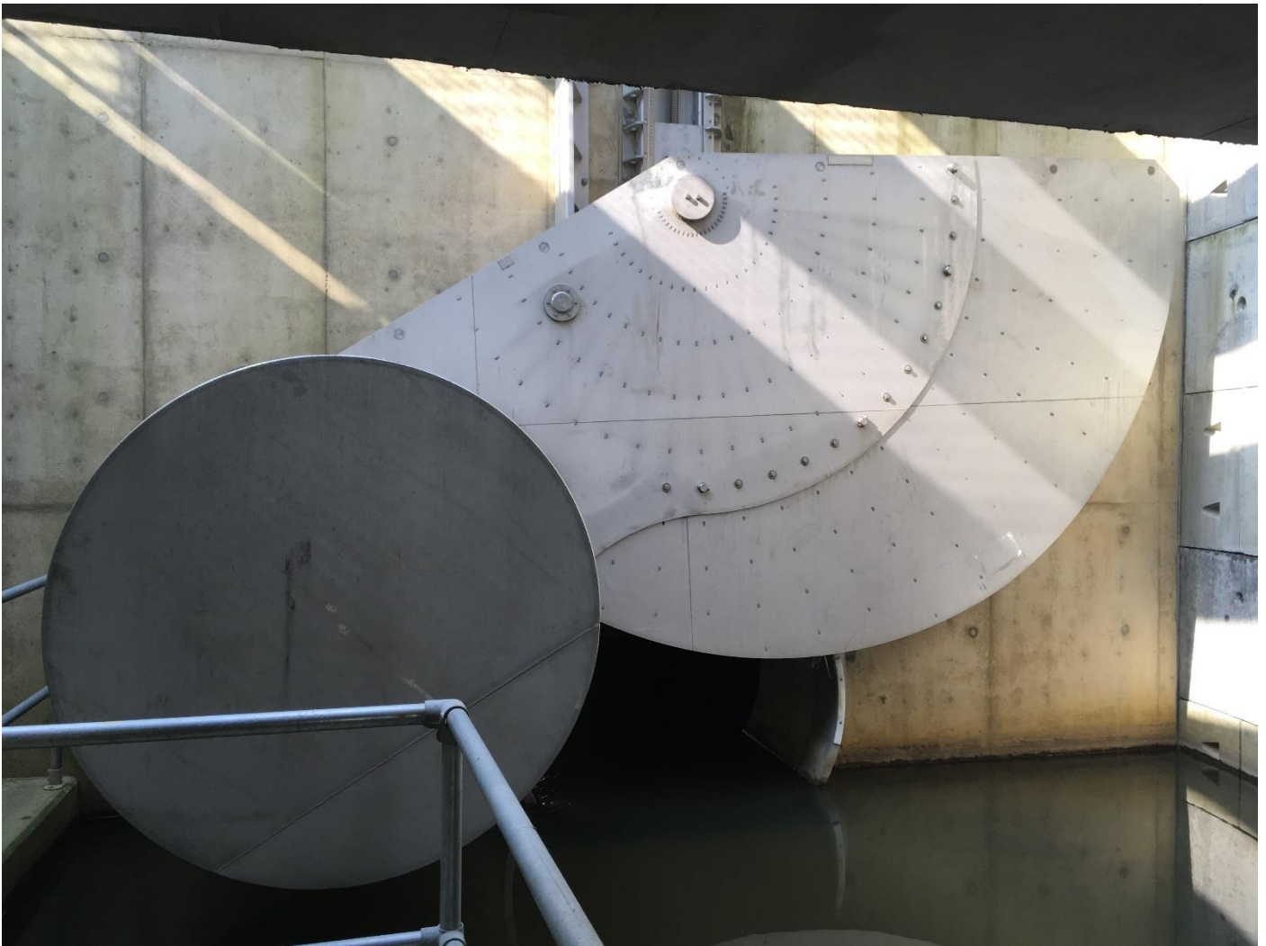
Photo 1: Hydroslide – rotates as water levels rise to restrict flows passing downstream
