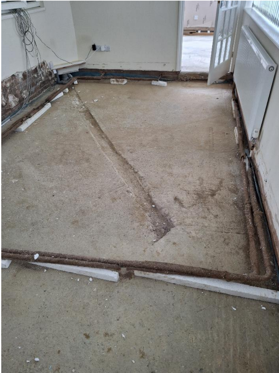
(Photograph 12.2 – Damages at [REDACTED])
