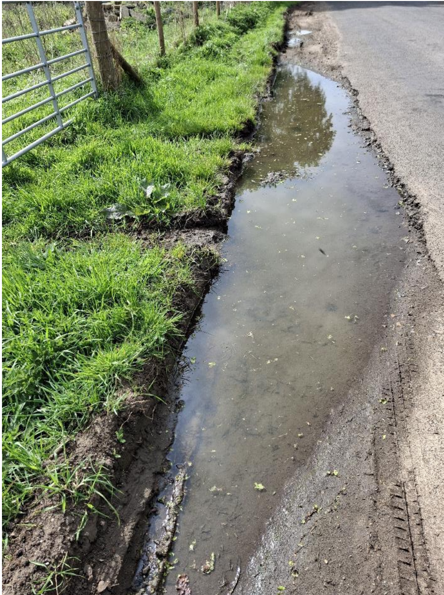
(Photograph 12.5 – Ponding on Hemingby Lane, [REDACTED]; facing south)
