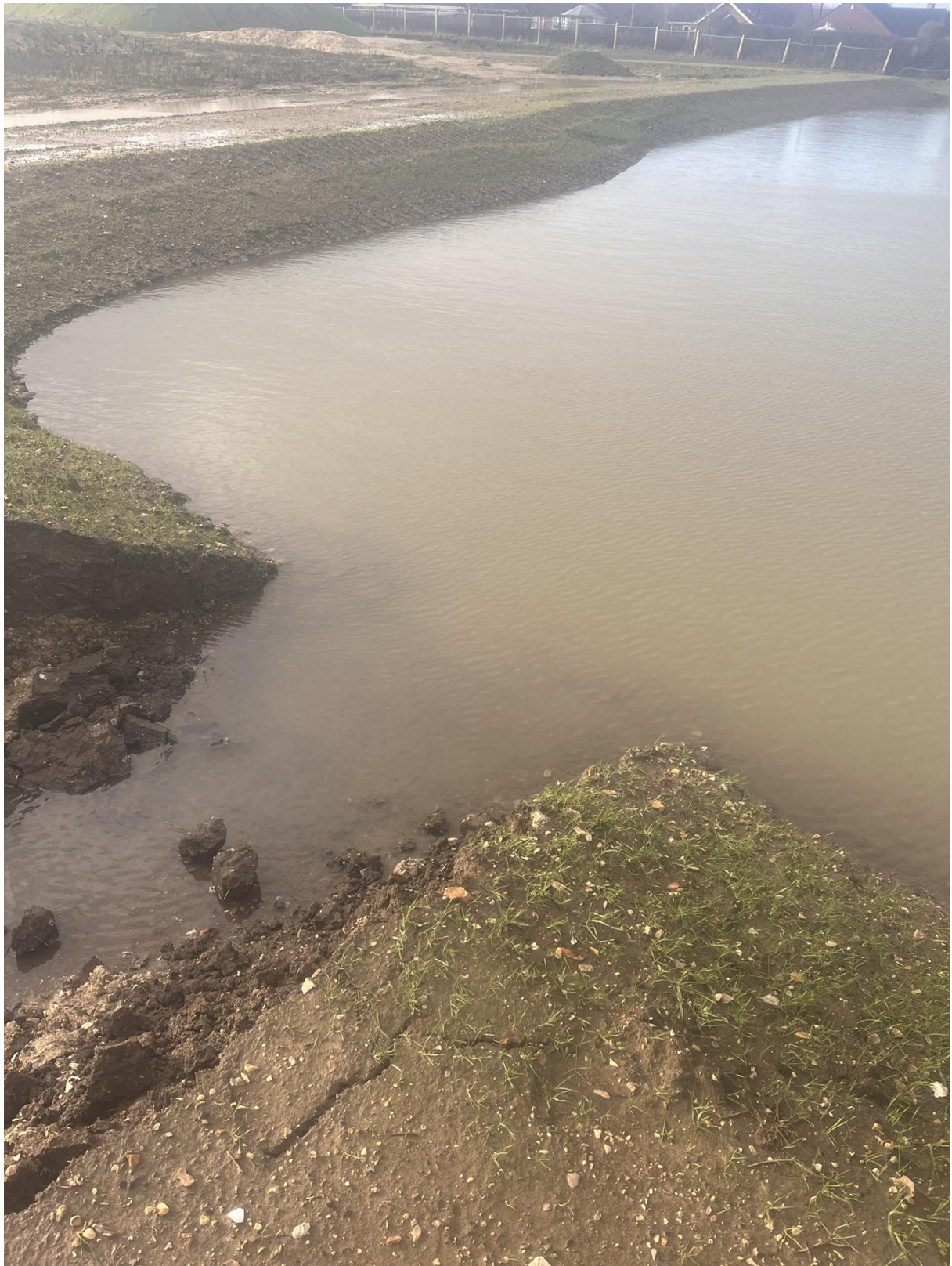
(Photograph 2.20 – Breach on Poppy Fields on-site attenuation pond)
