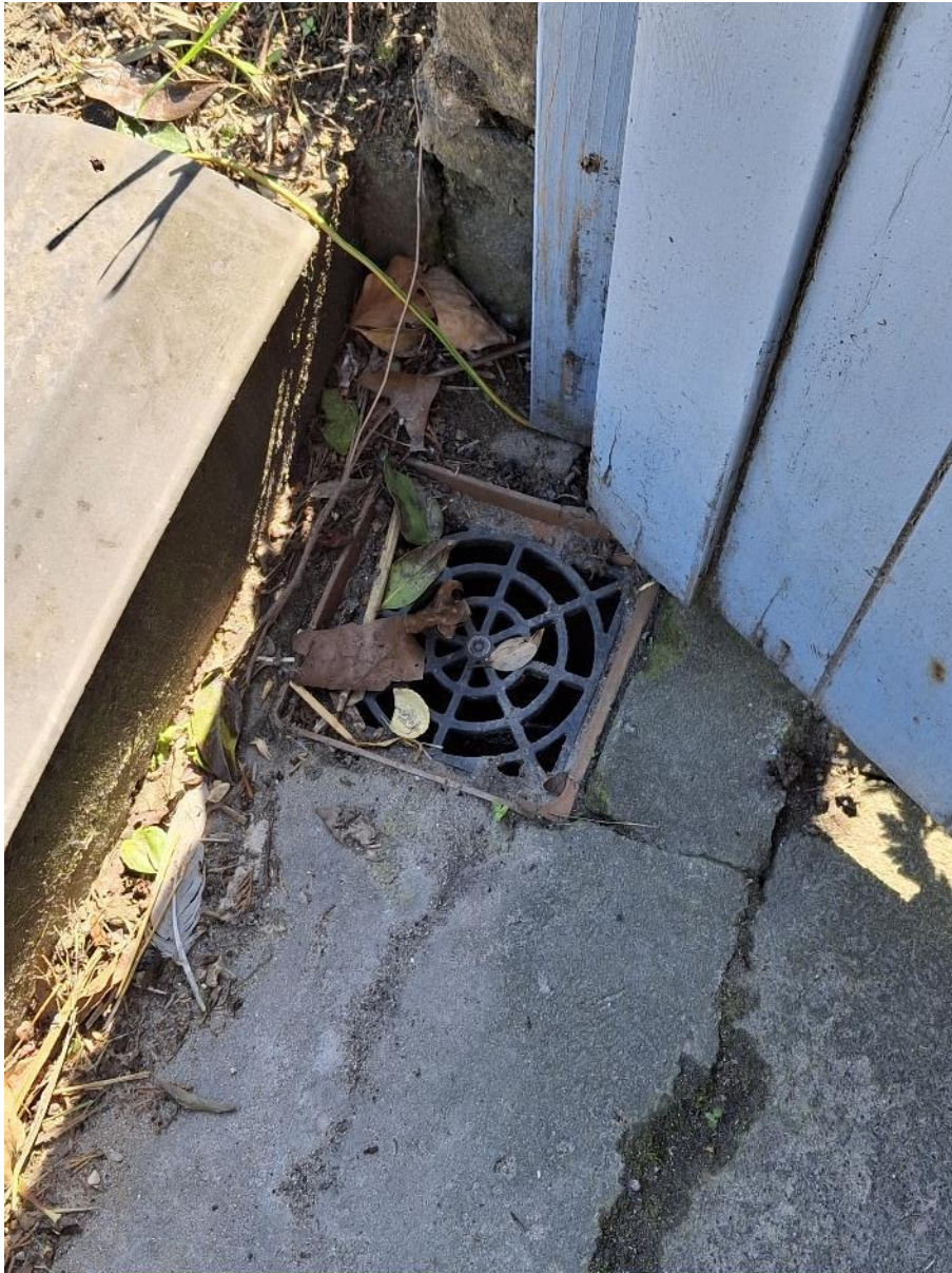
(Photograph 7.3 – Gully at the front door of [REDACTED])
