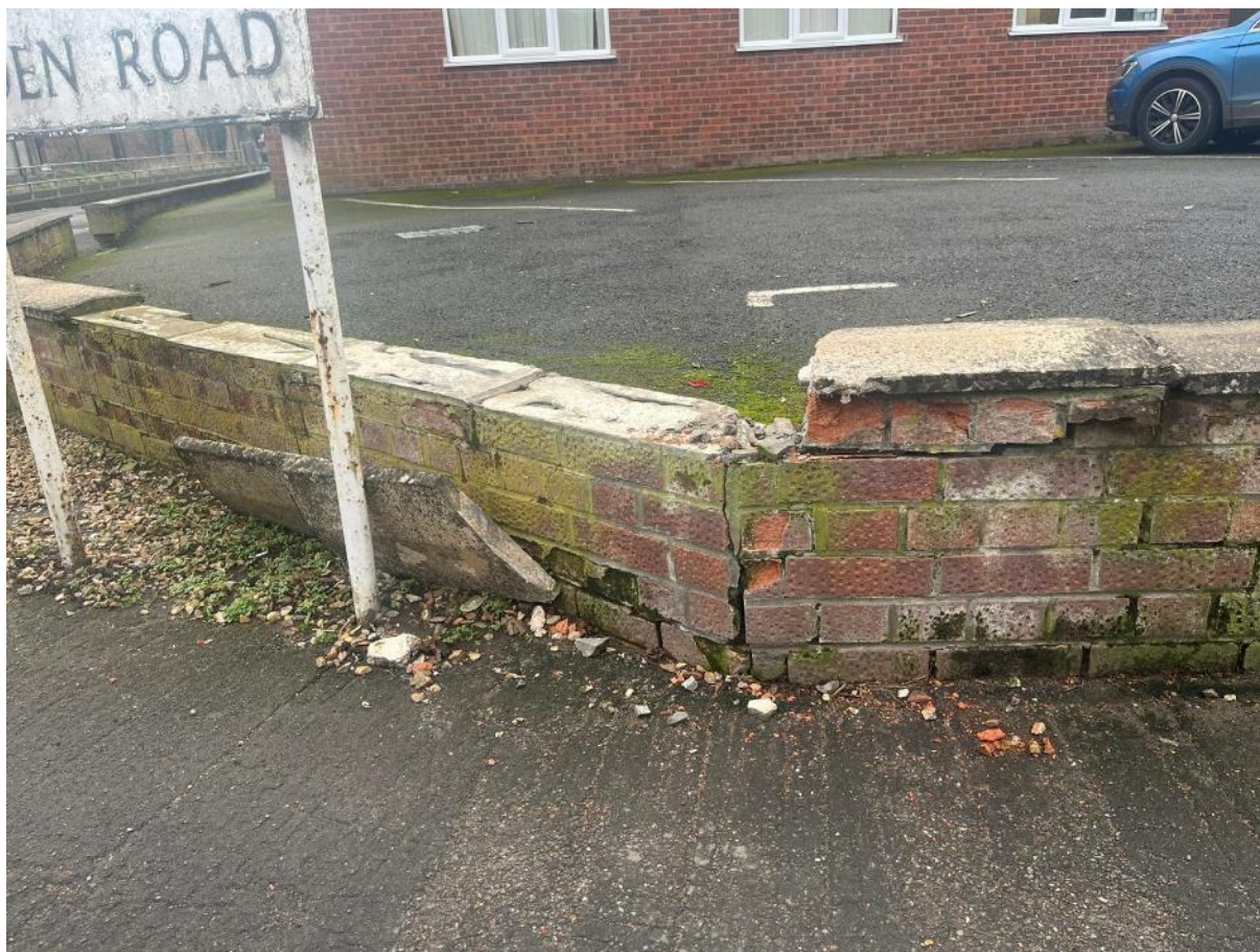
(Photograph 3.13– Broken wall caused by fluvial flows during Storm Babet, as provided by the manager at the [REDACTED] on Banks Street)
