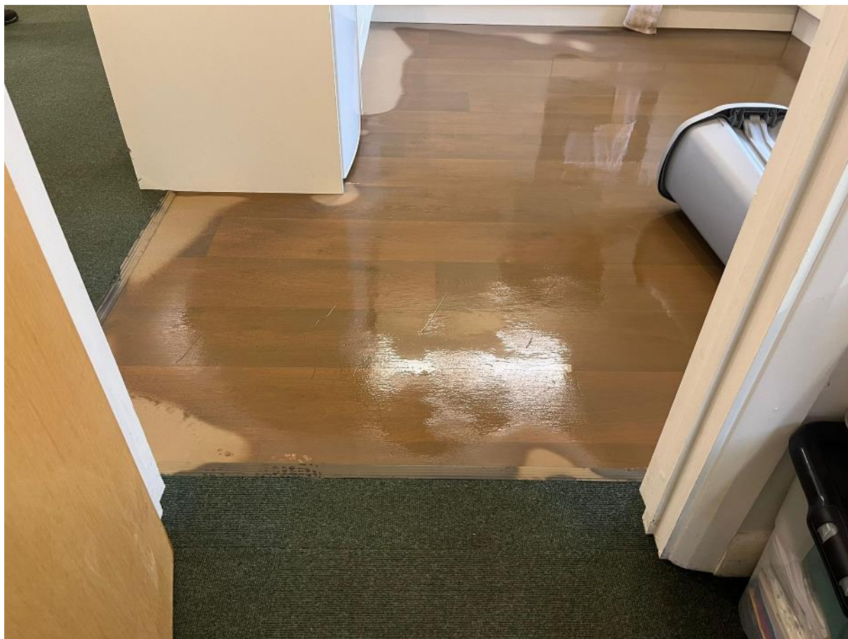
(Photograph 3.12 – Water inside [REDACTED] following Storm Babet.)
