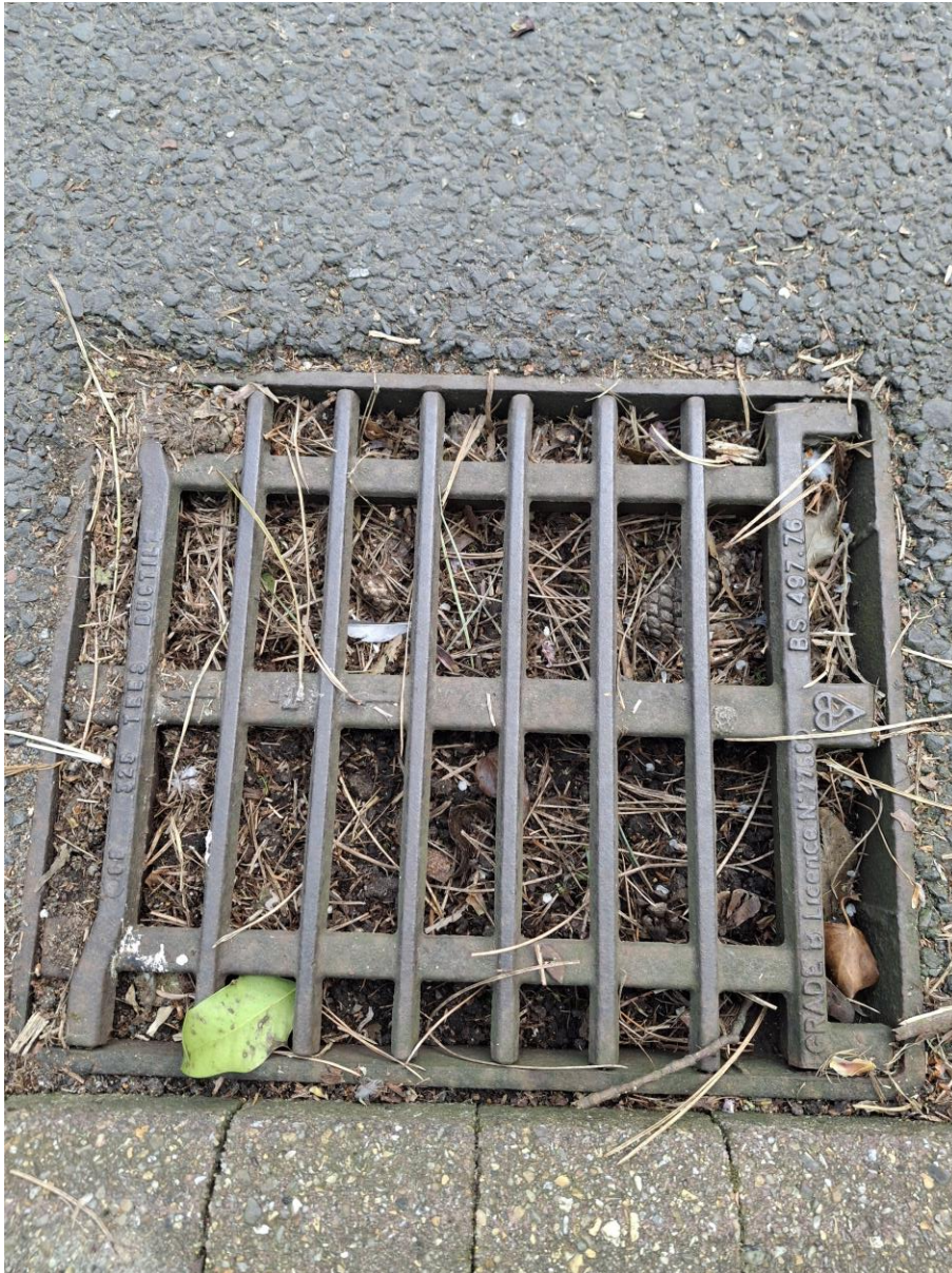
(Photograph 2.13 – Blocked gully on the entrance road to [REDACTED])
